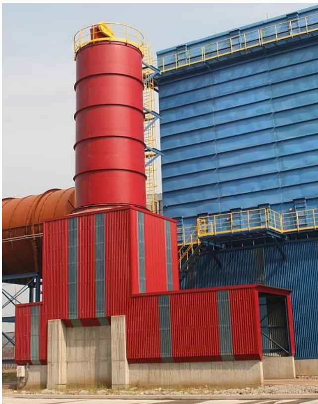
Dust collecting silo
