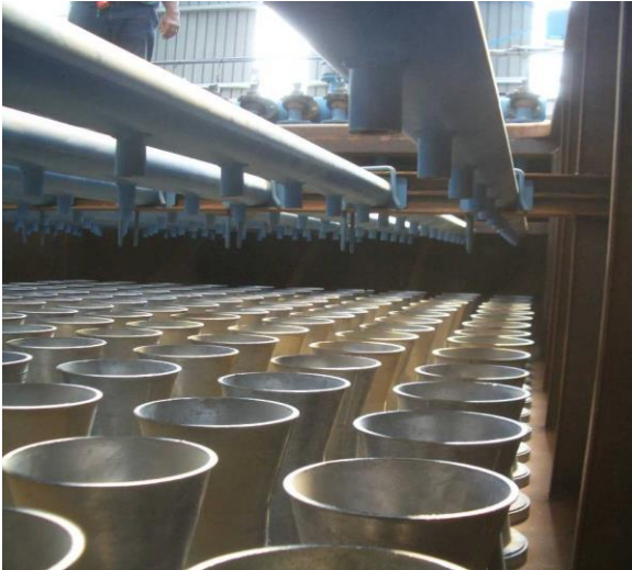
BAG FILTER – Internal view
