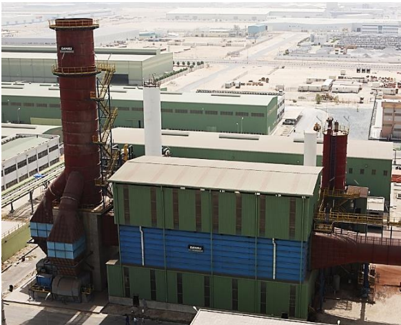
BAG FILTER – External view
