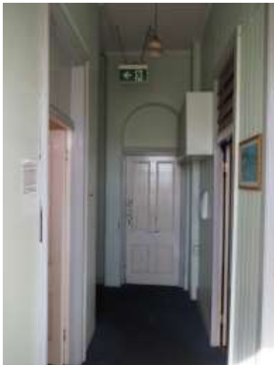
Some doors to the first floor and VJ ceilings, concealed with new sheeting to some of the front first floor bedrooms
