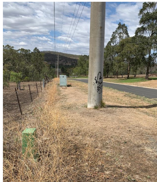
Figure 2: Southern Boundary St pole and transformer
