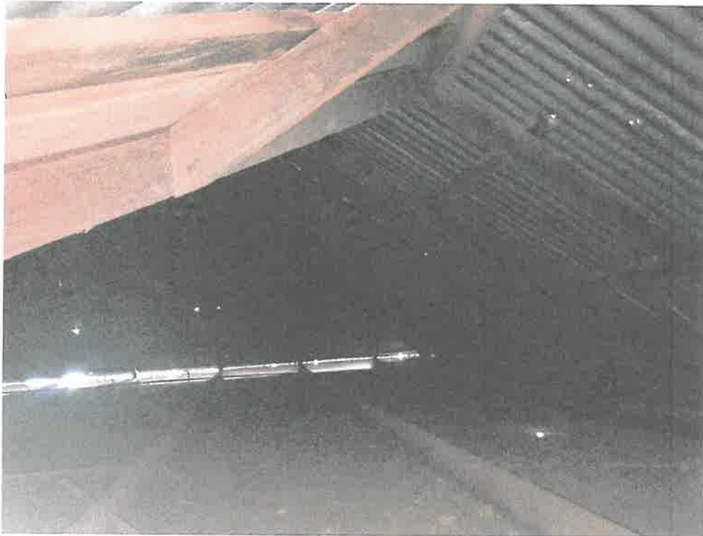
Photo 8 – View of Roof Cavity – Note no underpurlins or strutting to rafters, discontinuous roof battens, rust holes to roof sheeting.
