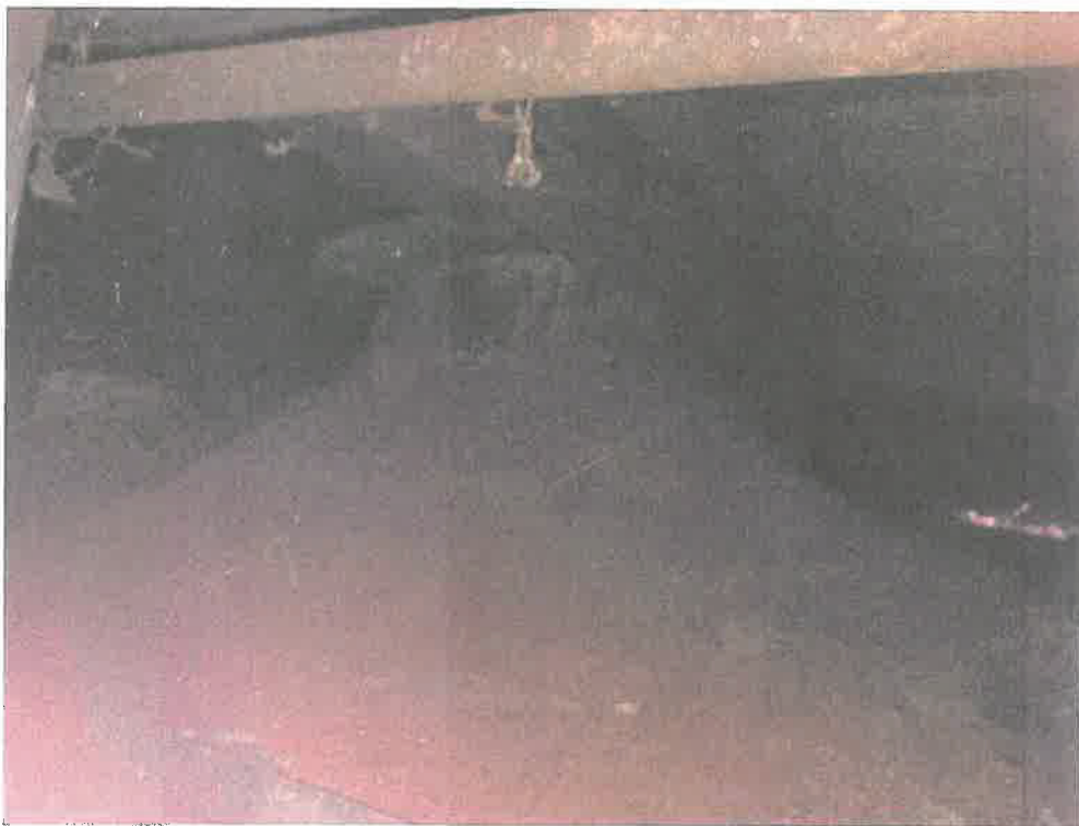
Photo 4 – Termite Mound under Residence.
