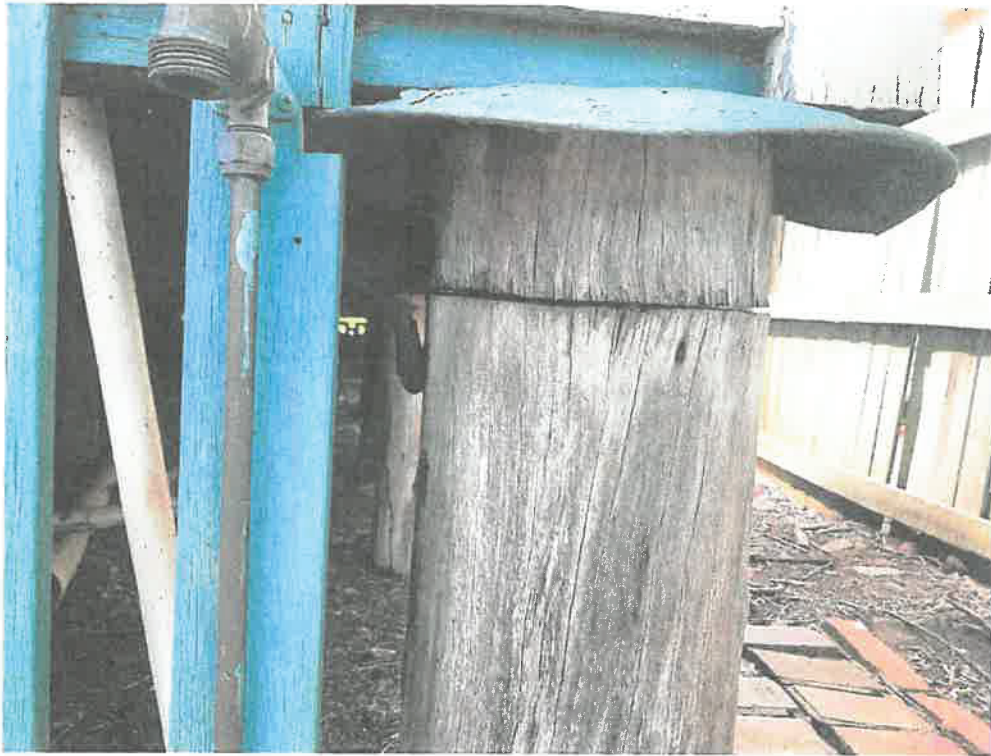
Photo 3 – Stump at front of residence
