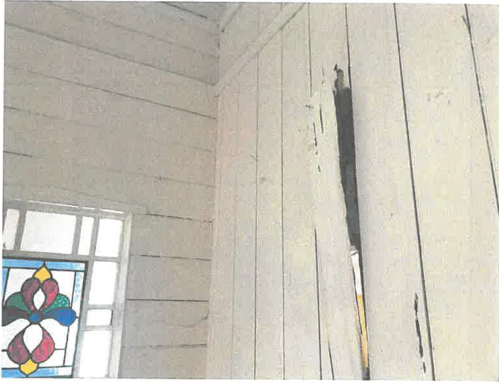
Photo 7 – Further termite damage to Internal Walls
