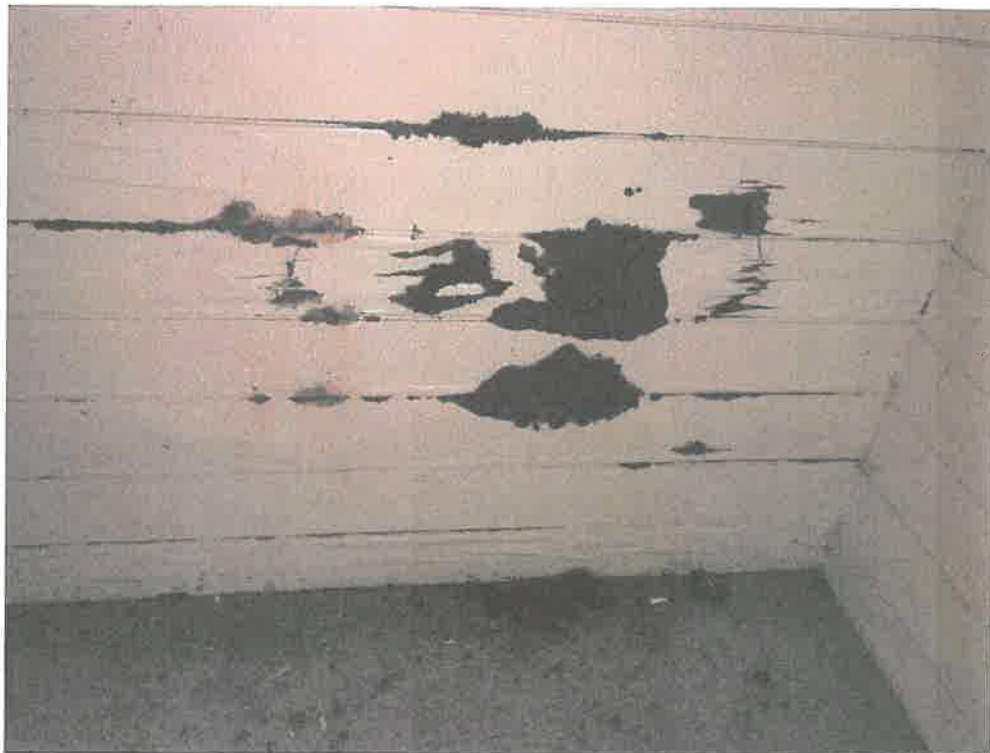
Photo 6 – Termite damage to Internal Walls.
