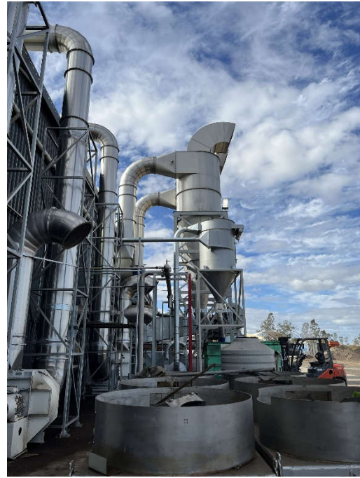
Fig 14 – External cyclones and air handling
