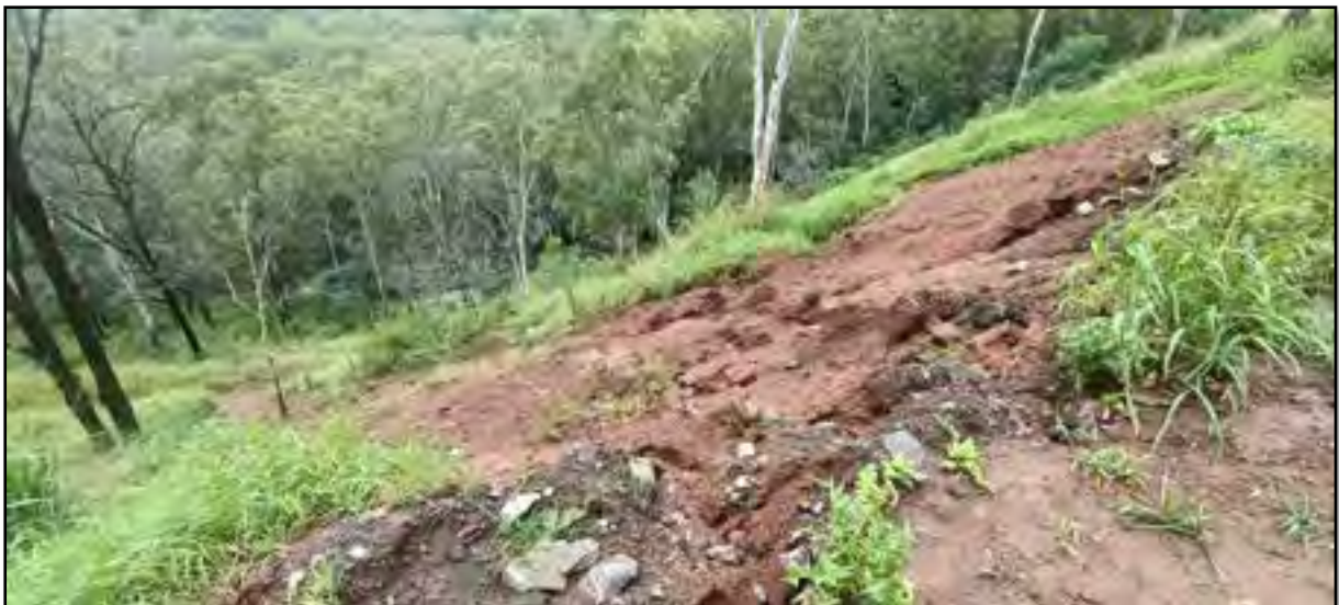
PLATE 3 – RECENT SLUMP ON OUTER EDGE
