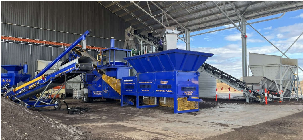
Fig 6 Blending and Pug Mill equipment
