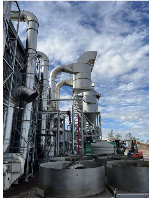
Fig 14 – External cyclones and air handling
