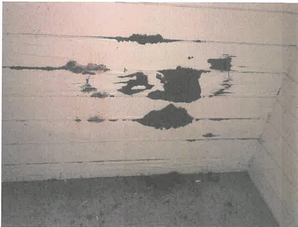
Photo 6 – Termite damage to Internal Walls.
