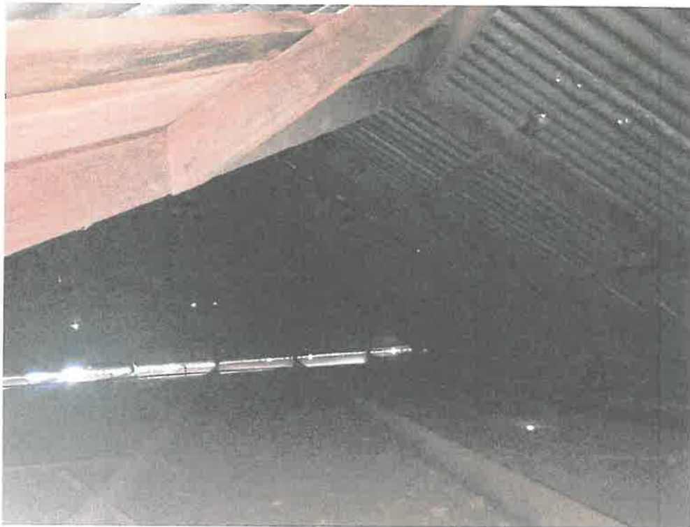
Photo 8 – View of Roof Cavity – Note no underpurlins or strutting to rafters, discontinuous roof battens, rust holes to roof sheeting.
