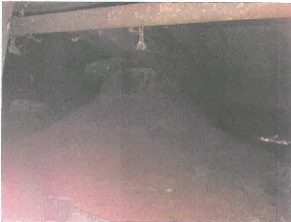
Photo 4 – Termite Mound under Residence.
