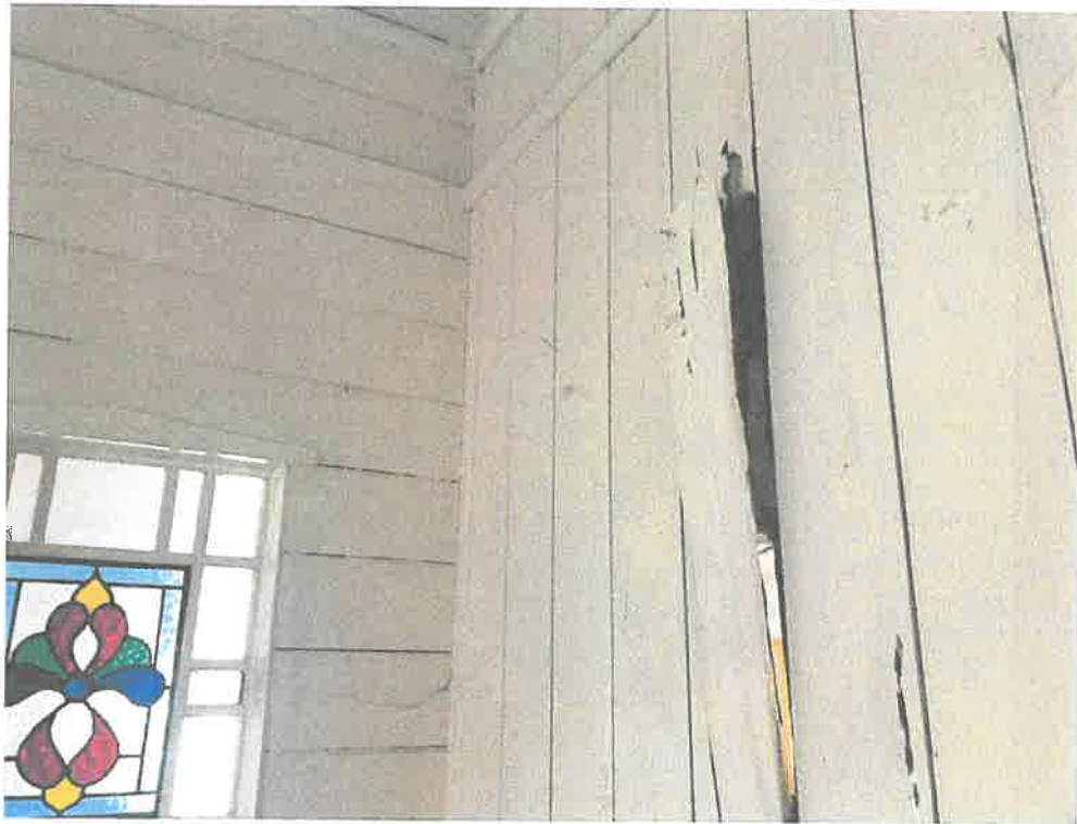
Photo 7 – Further termite damage to Internal Walls
