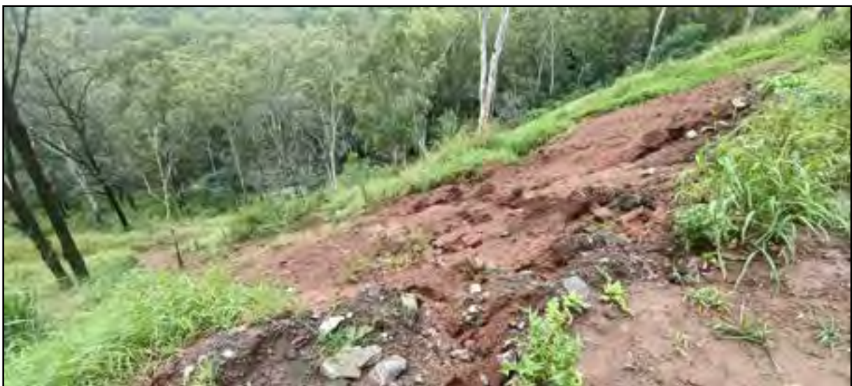
PLATE 3 – RECENT SLUMP ON OUTER EDGE
