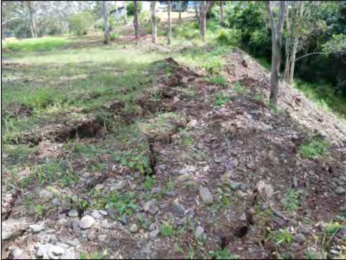
PLATE 6 – CRACKING OF FILL BATTER
