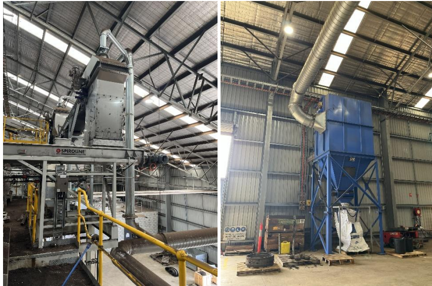
Organic manure processing - Dust extraction
