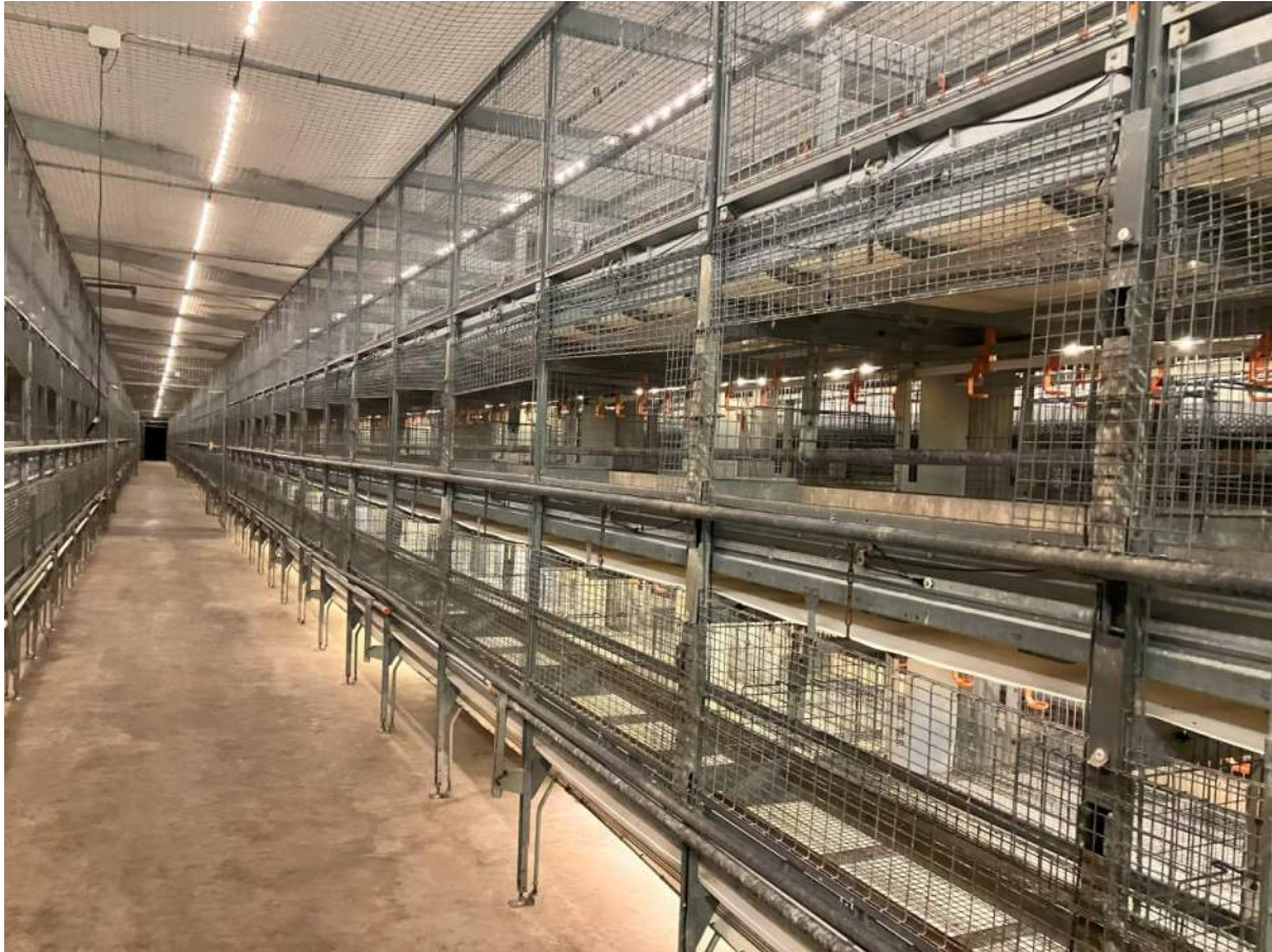
Photograph 2 – Aviary systems will be in place along the length of the sheds
